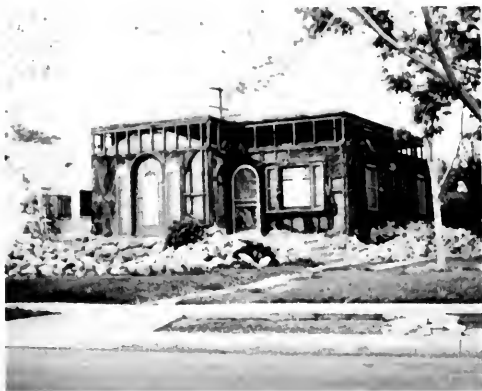
Photo 7. Older wood frame dwelling with unanchored stone veneer, in San Fernando.
